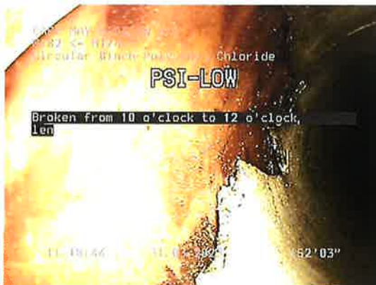
M182_M174_3312023 120938 PM_B_58.jpg, 00:08:59, 152.28ft Broken from 10 o'clock to 12 o'clock, length: 15inch
