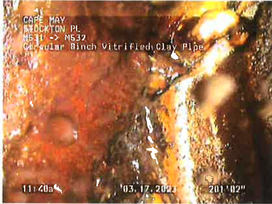
M531_M532_11192022 34432 AM_IR_25.jpg, 00:30:01, 201.18ft Infiltration Runner from 8 o'clock to 4 o'clock, within 8 inch
