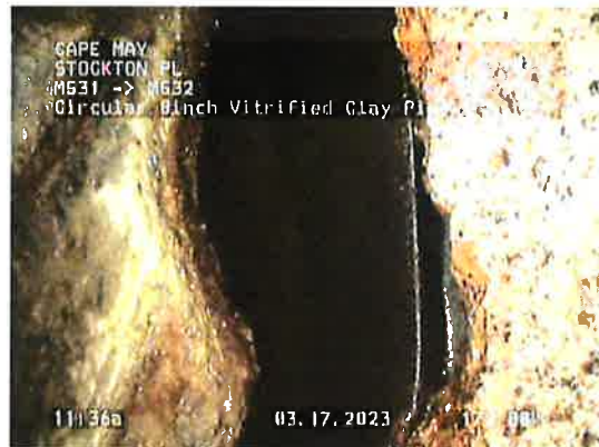
M531_M532_11192022 34432 AM_B_24.jpg, 00:25:58, 172.02ft Broken from 8 o'clock to 4 o'clock, within 8 inch
