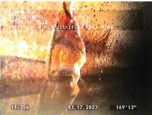
M531_M532_11192022 34432 AM_FC_23.jpg, 00:25:35, 169.99ft Fracture Circumferential from 8 o'clock to 4 o'clock, within 8
