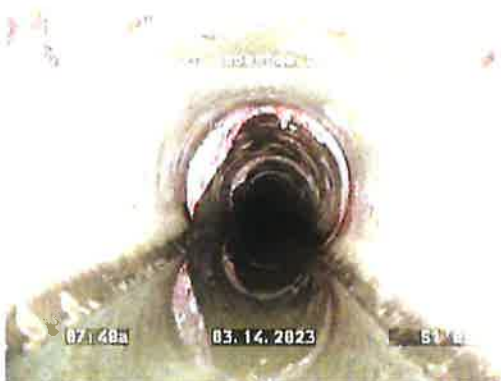
M236_M233_3142023 81806 AM_DAE_15.jpg, 00:09:35, 51.23ft Deposits Attached Encrustation, 5% of cross sectional area
