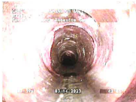
M236_M233_3142023 81806 AM_DAE_14.jpg, 00:08:21, 42.42ft Deposits Attached Encrustation, 5% of cross sectional area
