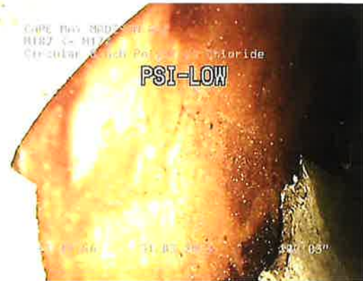
M182_M174_3312023 120938 PM_B_57.jpg, 00:08:59, 152.28ft Broken from 10 o'clock to 12 o'clock, length: 15inch
