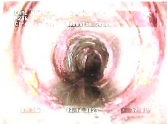
M236_M233_3142023 81806 AM_DAE_13.jpg, 00:05:16, 39.38ft Deposits Attached Encrustation, 5% of cross sectional area
