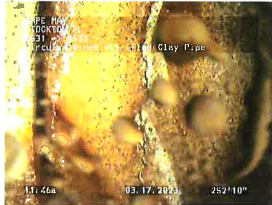
M531_M532_11192022 34432 AM_B_26.jpg, 00:35:05, 252.91ft Broken from 7 o'clock to 11 o'clock, within 8 inch
