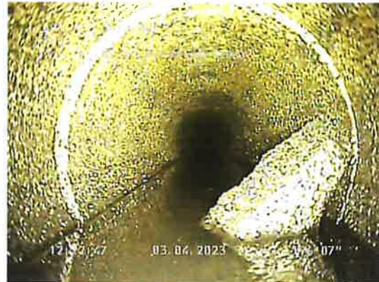
M350_M349_432023 11321 PM_OBB_102.jpg, 00:10:00, 196.73ft Obstruction Brick or Masonry, 5% of cross sectional area from
