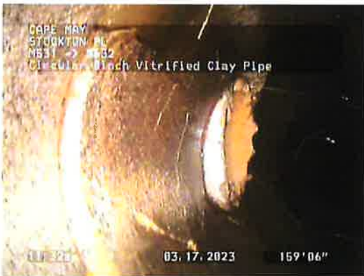
M531_M532_11192022 34432 AM_B_21.jpg, 00:23:07, 159.97ft Broken from 12 o'clock to 12 o'clock, within 8 inch
