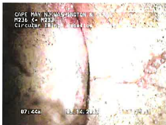
M236_M233_3142023 81806 AM_CL_16.jpg, 00:12:08, 71.08ft Crack Longitudinal at 1 o'clock, within 8 inch
