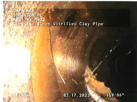
M531_M532_11192022 34432 AM_B_20.jpg, 00:23:07, 159.97ft Broken from 12 o'clock to 12 o'clock, within 8 inch
