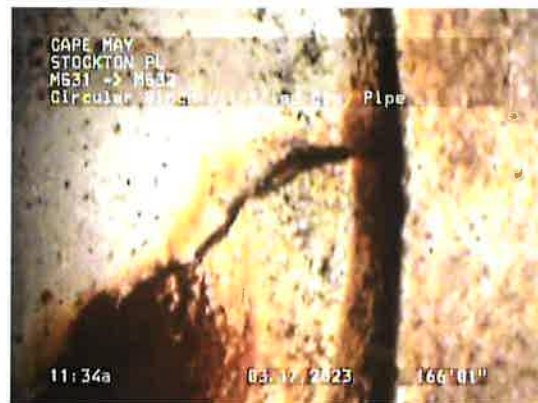
M531_M532_11192022 34432 AM_FC_22.jpg, 00:24:22, 166.15ft Fracture Circumferential from 12 o'clock to 4 o'clock, within 8
