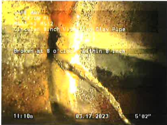
M531_M532_11192022 34432 AM_B_19.jpg, 00:06:36, 5.16ft Broken at 8 o'clock, within 8 inch
