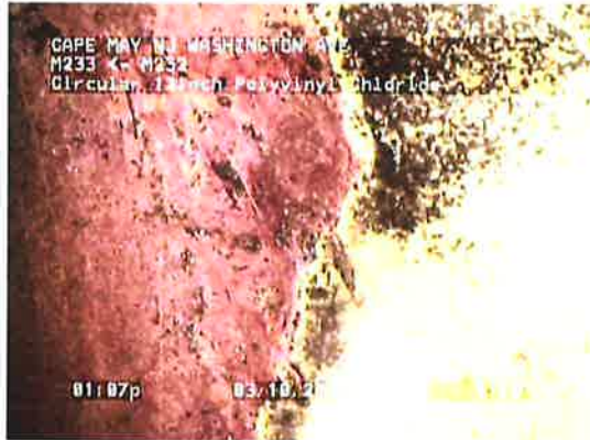
M233_M232_3102023 125258 PM_IRJ_113.jpg, 00:02:18, 5.97ft Infiltration Runner Joint at 2 o'clock, within 8 inch
